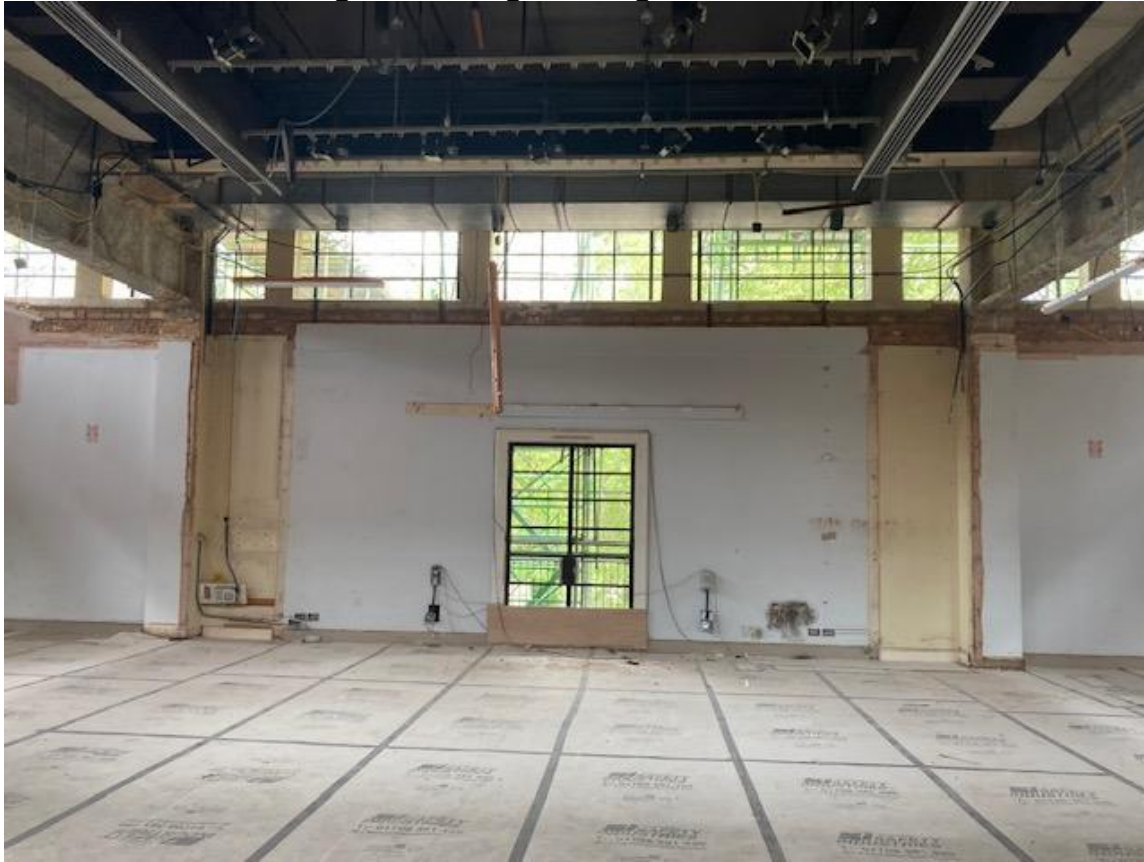
Figure 5: Middlesex Suite – Internal works for re-instating high-level windows and restoring central high ceilings.
